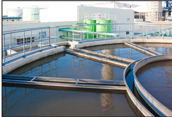
Condition of 1st tank coated with ARC 858 and ARC S1PW after 11 years in service.
